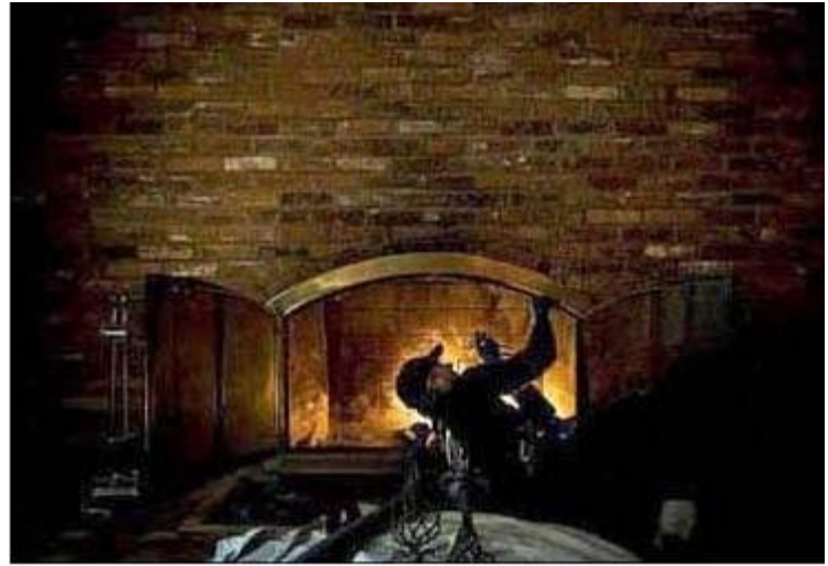
Walter Kerr replaces the handle of a fireplace flue. Homeowners should have their chimneys inspected annually.
